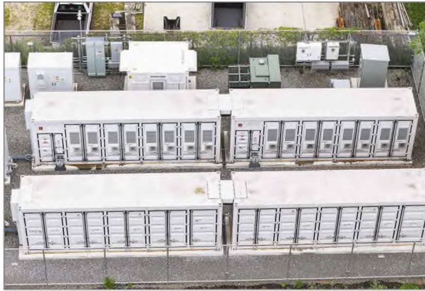
Battery storage units in Patchogue. There are 11 lithium-ion battery storage plants proposed for Suffolk.
